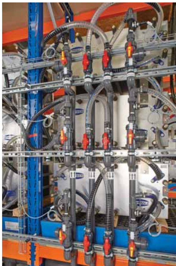
Figure 8. Piping and stacks of a 2 MW/20 MWh vanadium redox flow battery at Fraunhofer ICT
